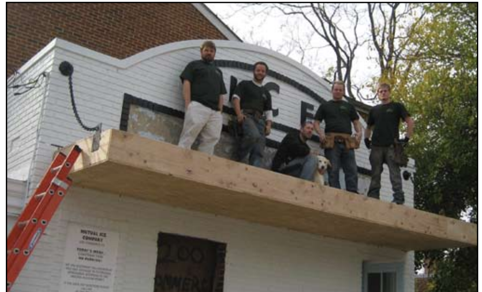
The crew of Greensaw Design & Build on the scene of the Ice House project in historic Alexandria, Va. Photo courtesy of Greensaw Design & Build
